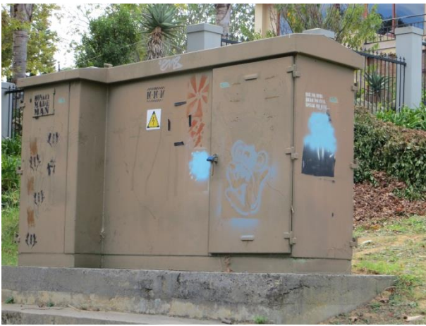
Figure 17 Illegal Posters on public infrastructure
