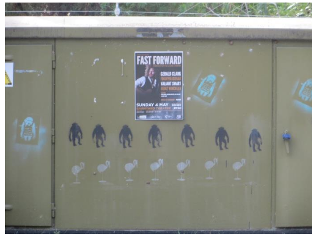
Figure 18 Illegal Posters on public infrastructure
