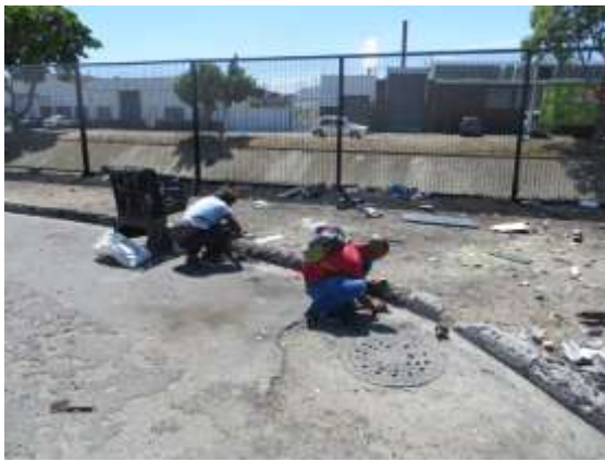
Figure 48 Public infrastructure in a state of disrepair – in many cases due to illegal processing of scrap on the sidewalks
