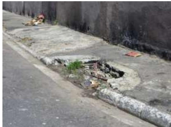
Figure 45 manhole on sidewalk without proper cover
