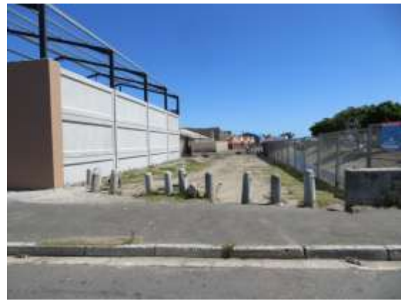
Figure 49 Broken infrastructure such as these walkways and bollards shows neglect of certain aspects.
