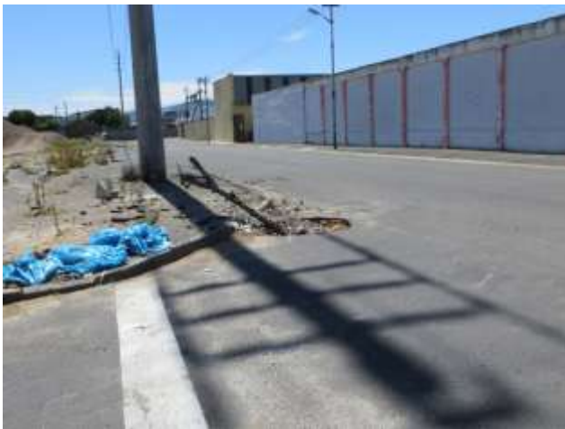
Figure 53 Storm water drains are blocked or completely absent due to poor road maintenance
