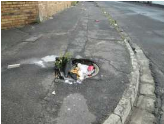
Figure 46 Open manhole on sidewalk
