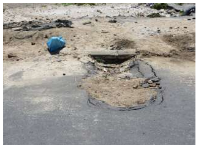
Figure 52 Some road surfaces, kerbs and gutters are badly maintained
