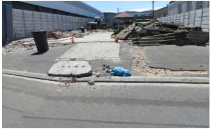
Figure 43 Poor sidewalk surface
