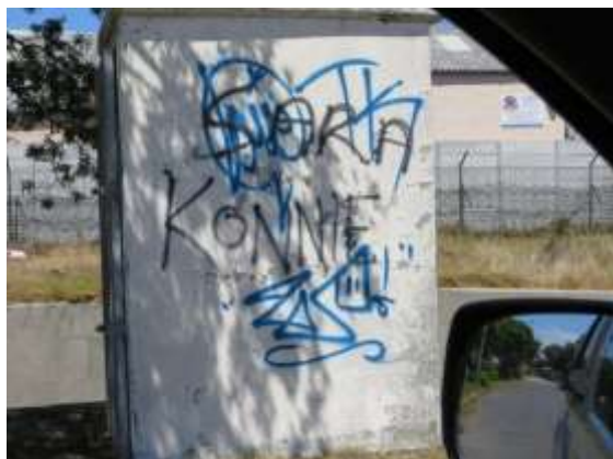
Figure 23 Graffiti on a building
