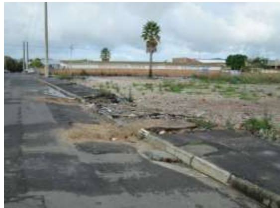
Figure 47 Very poor sidewalk conditions
