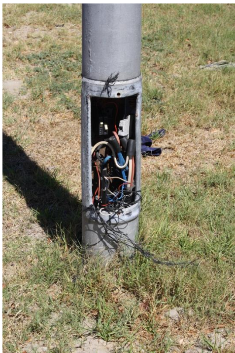
Figure 44 Public infrastructure in a state of disrepair
