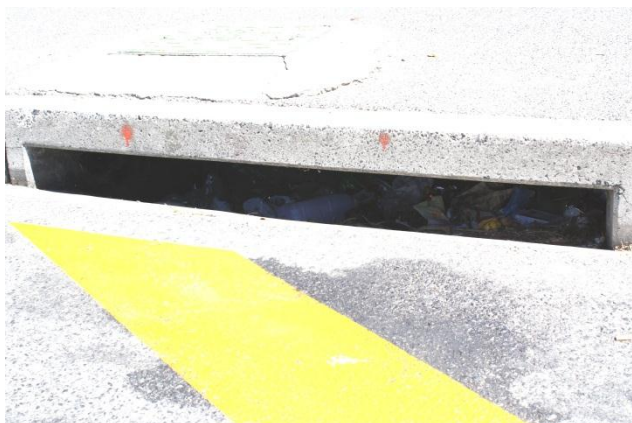
Figure 46 Some sidewalks and roads show kerb inlet and drains blocked due to litter
