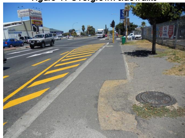
Figure 43 Sidewalk maintenance not completed
