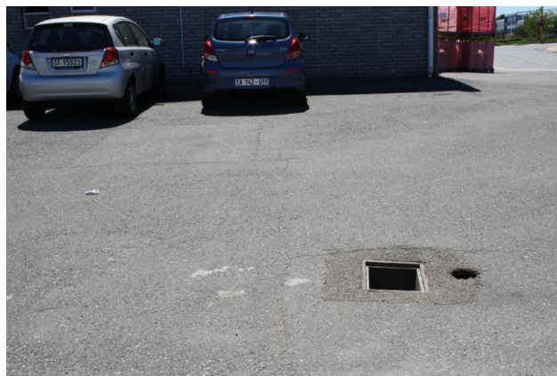
Figure 47 Some road surfaces and parking areas are without manhole covers
