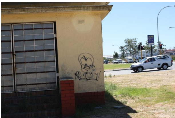
Figure 22 Graffiti on a building
