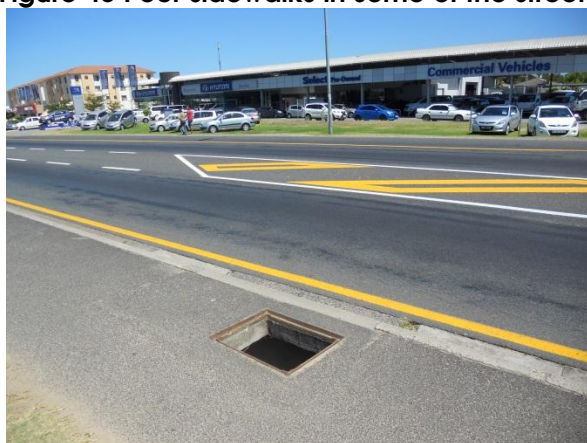
Figure 42 manhole on sidewalk without proper cover
